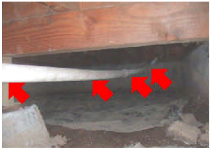
Missing supports for sump discharge line
