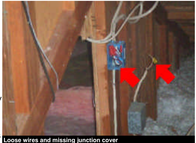
Loose wires and missing junction cover
